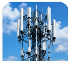
Communications System Testing
