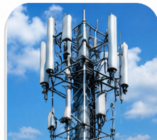
Communications System Testing
