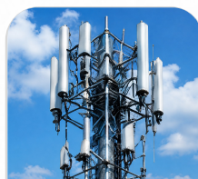
Communications System Testing
