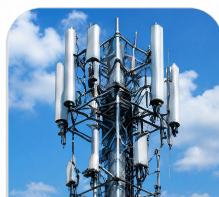
Communications System Testing
